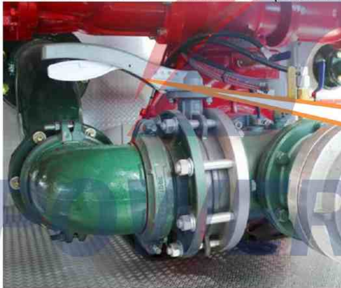
Turn off the Outlet Valve of Tank
