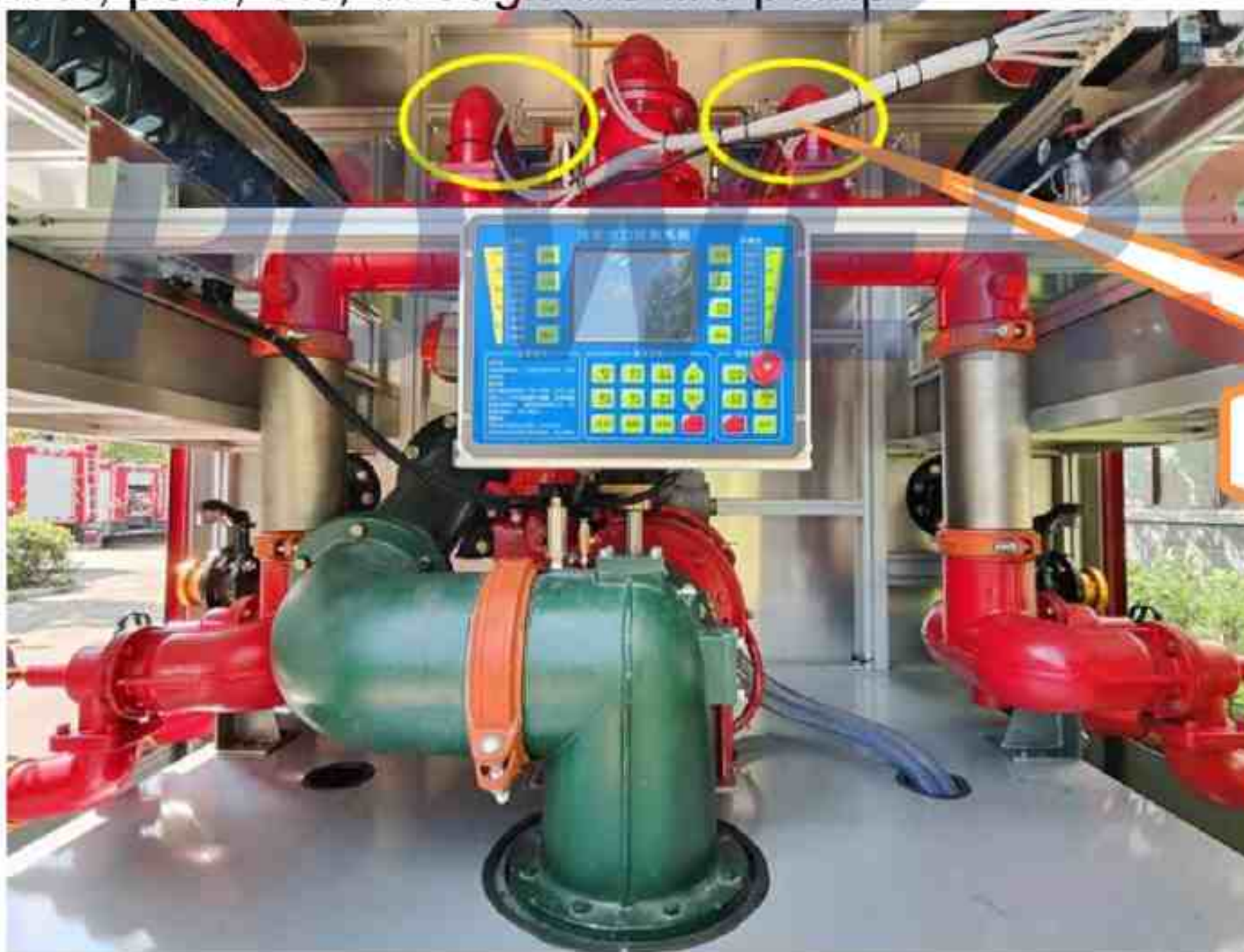
Water Inlet Control Valve:
